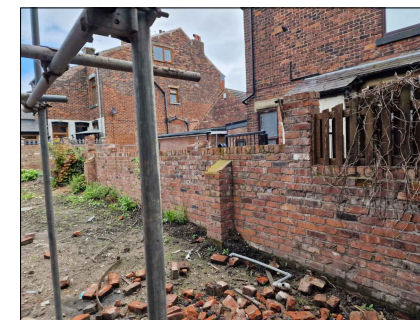
Existing boundary wall to 104 to be reinstated. Brick piers rebuilt where necessary and fence panels installed between piers to match existing
